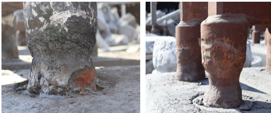
Figure 17. Corroded anode stubs before and after cleaning oxidized layer.
